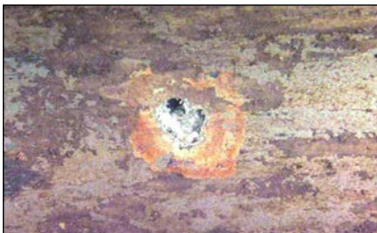
Figure 4. Manganese-induced pitting in stainless steel tube.
