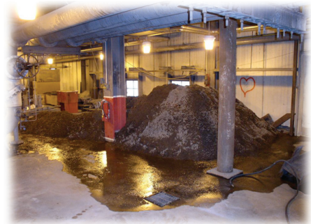
Calcium carbonate deposits removed from condenser. Photo: Courtesy of Conco Systems, Inc.
